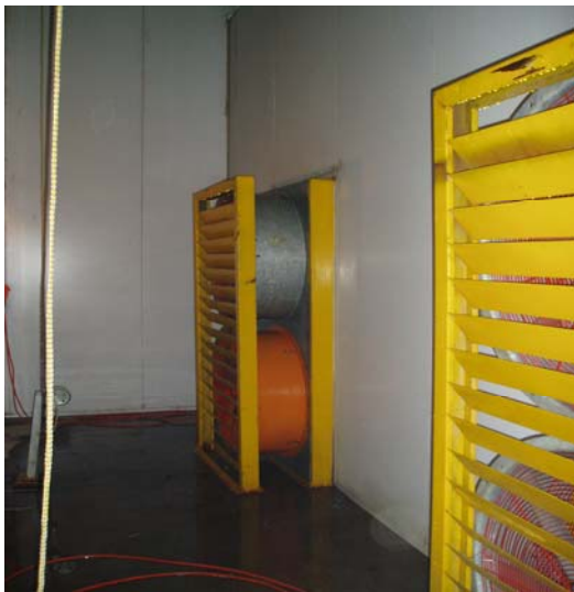
Fig. 1; Forced air fans from behind plenum wall
