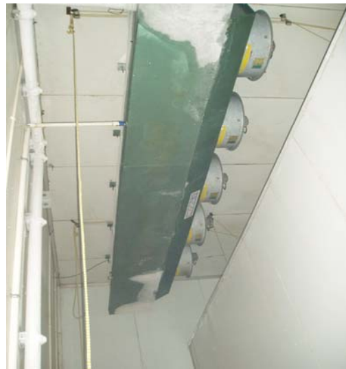
Fig 2; Cooling fan bank at top of plenum wall
