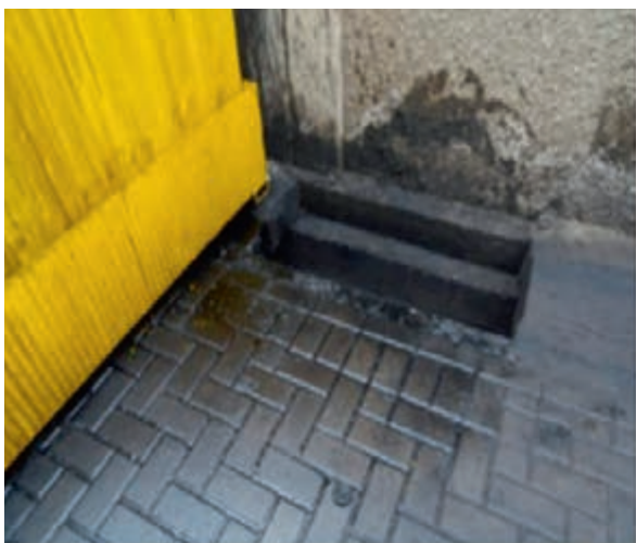
c. waste oil spilled into gutter
