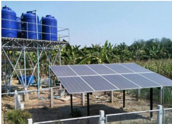
Solar water pump
