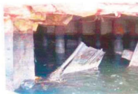
Figure 31 Damaged portion of TCIPC quay wall (2006) before rehabilitation
