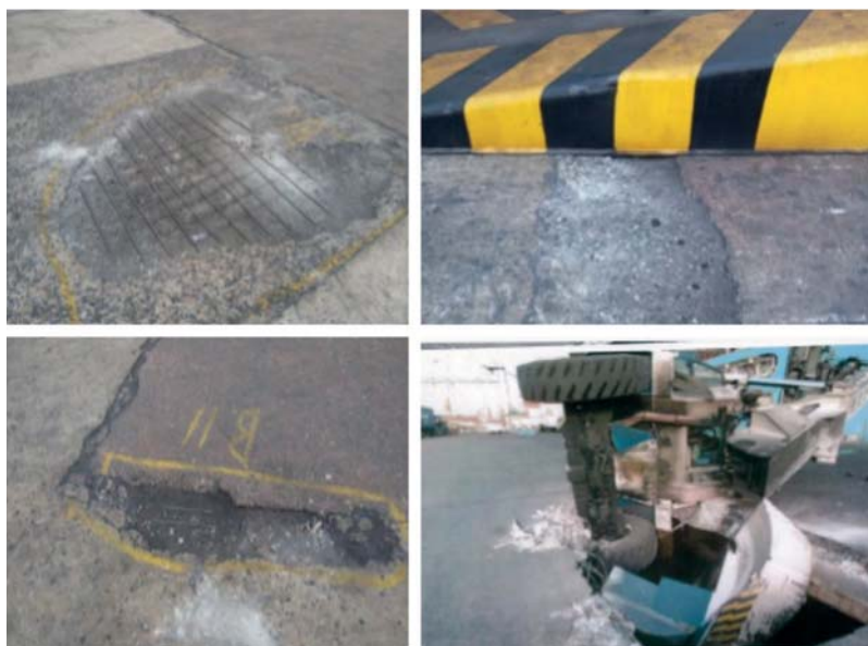
Figure 32 Damaged portion of TCIPC quay apron (2017) after rehabilitation
