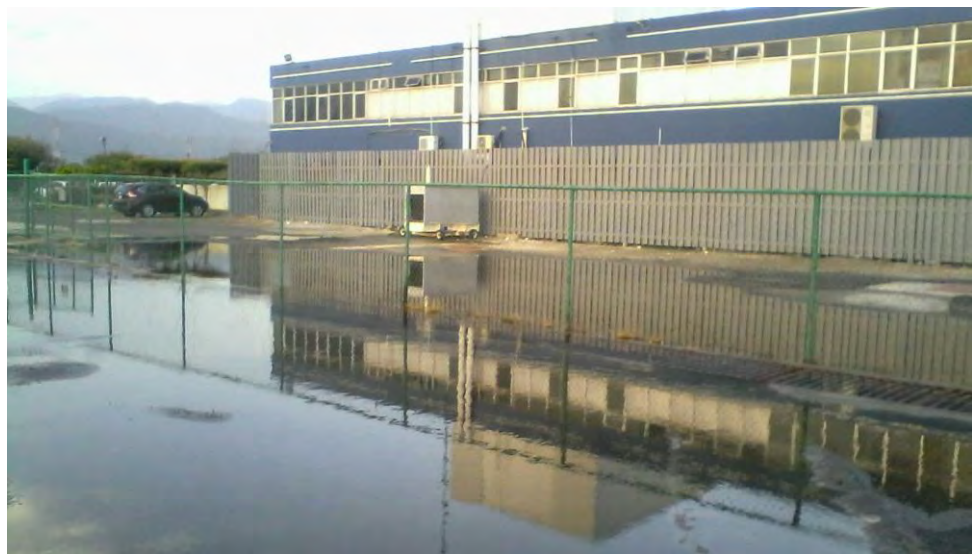
Figure 5.2 Flooding of area behind Administration Building
