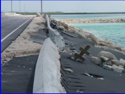
North to Middle Caicos Causeway following TS Hanna and Hurricane Ike, 2008
