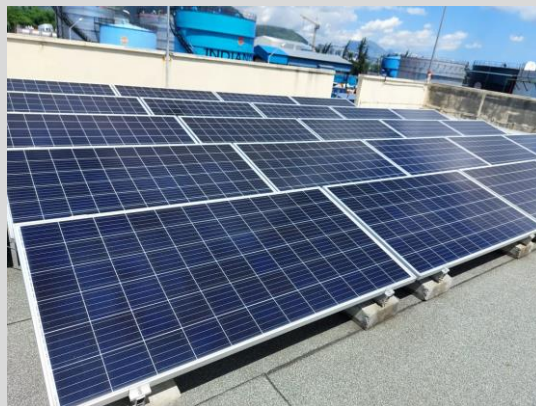
Solar PV Installations at Oil Jetty Port Louis Harbour, Mauritius
