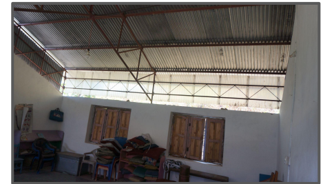
Fig: Roofing with no underlying layering
