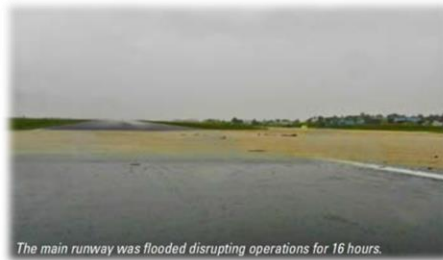
The main runway was flooded disrupting operations for 16 hours.
