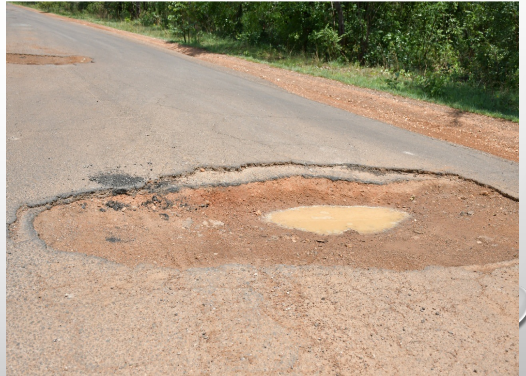
EXTENT OF POTHOLE
