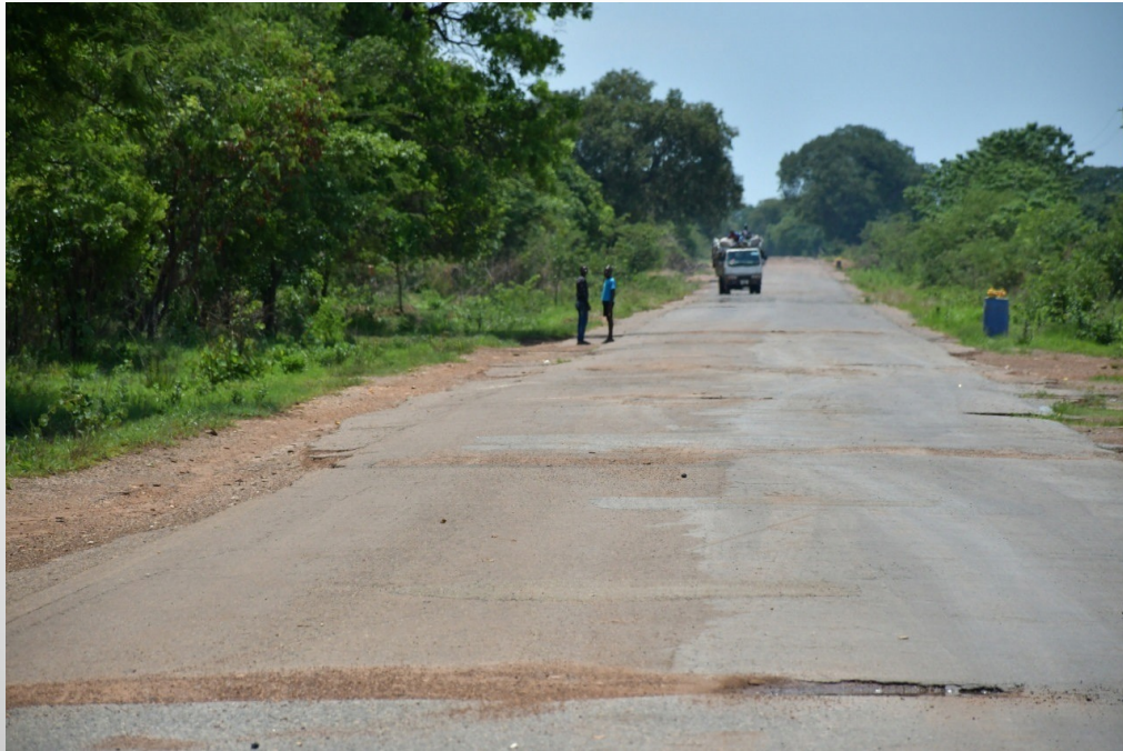
POTHOLE CUT ACROSS ROAD
