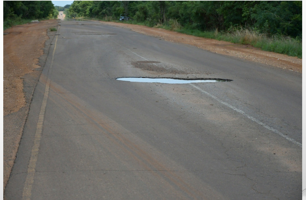
POTHOLE IN MIDDLE OF ROAD
