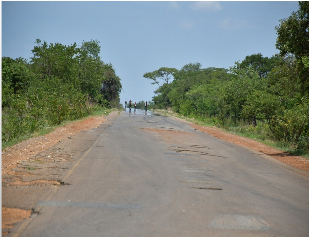
MULTIPLE POTHOLES ALONG ROAD SECTION
