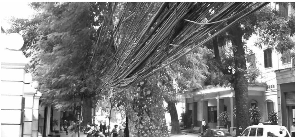
Figure 3.5: Electricity connections in Hanoi
