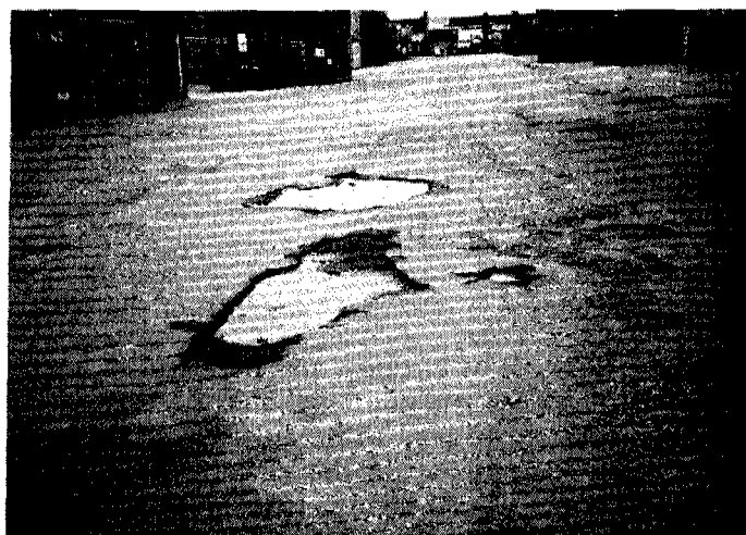
Damage from heavy container handling equipment
